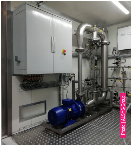
Filtration skid realization
